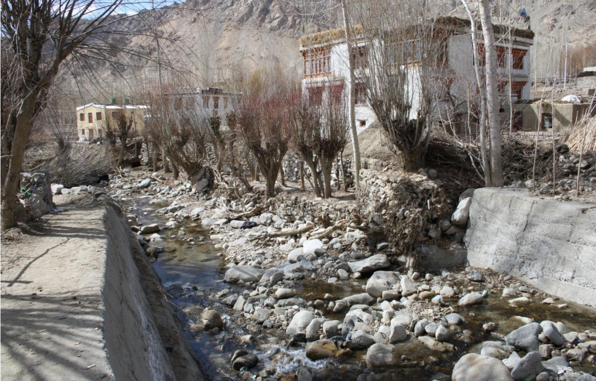
Figure 7.3. View of the river in Chanspa, one of the upper areas of Leh, and the embankments damaged by the floods of 2010 (Le Masson, 2011)
