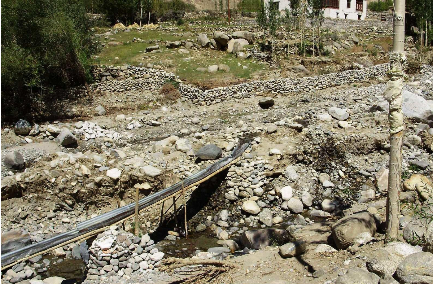
Figure 5.6. Repairs undertaken along the river stream in Saboo using meatl steel (Le Masson, 2011)
