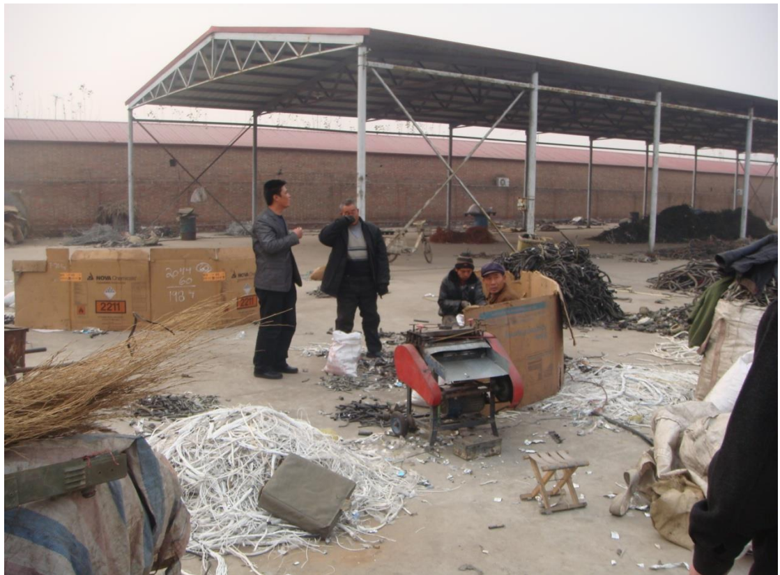
Figure 5.5 The local workers are stripping cable under unsafe and poor work condition.
