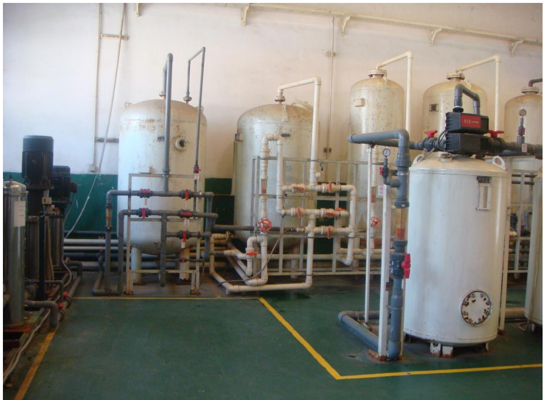
Figure 5.3 The second water recycle system of Shenyi manufacturing plant.
