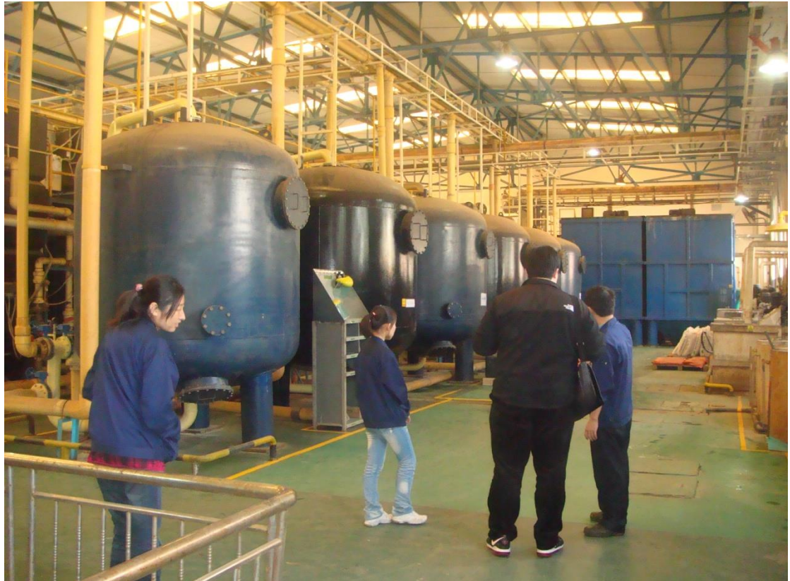
Figure 5.4 The third and newest water recycle system of Shenyi manufacturing plant.
