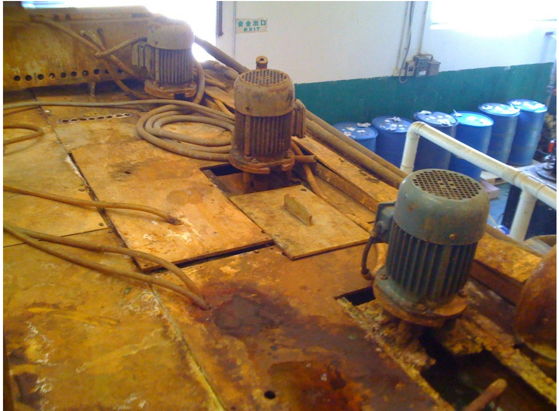
Figure 5.2 The first and oldest water recycle system of Shenyi manufacturing plant.
