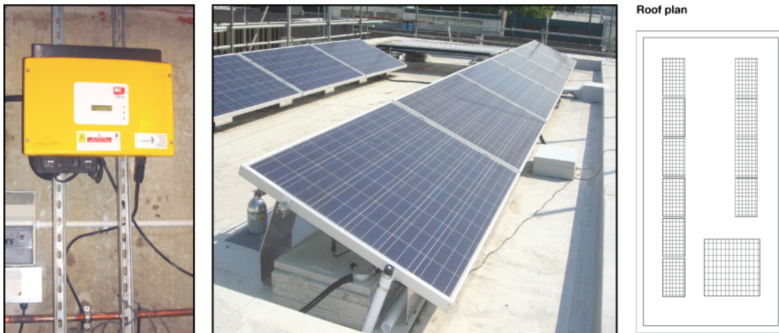
Figure 5.35 Photovoltaic panels on the roof and the inverter in the plant room.
