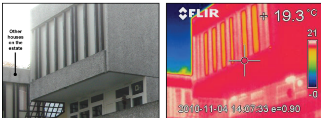
Figure 5.5 Thermal image of the asbestos wall and overhanging bedroom.
