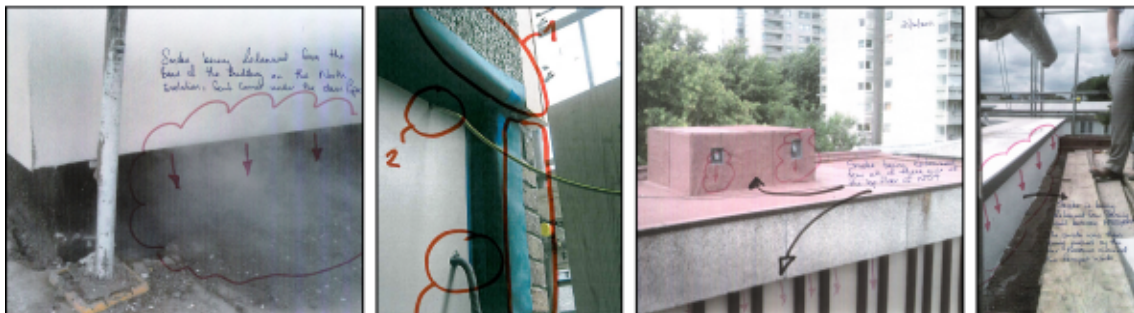
Figure 5.41 Main sources of air leakage identified during smoke testing.
