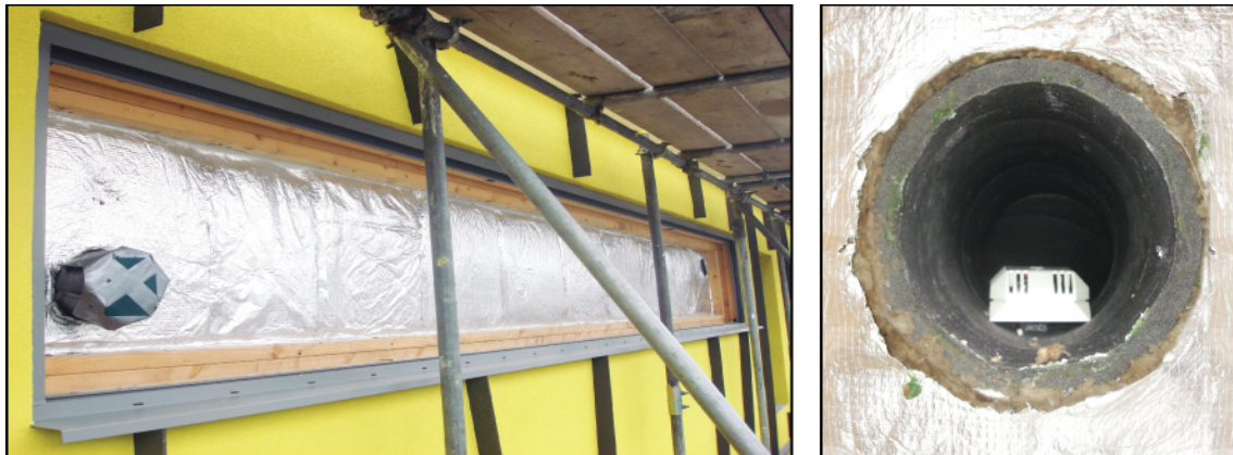
Figure 6.6 Collector showing the foil backed insulation and thermistor in the outlet duct.
