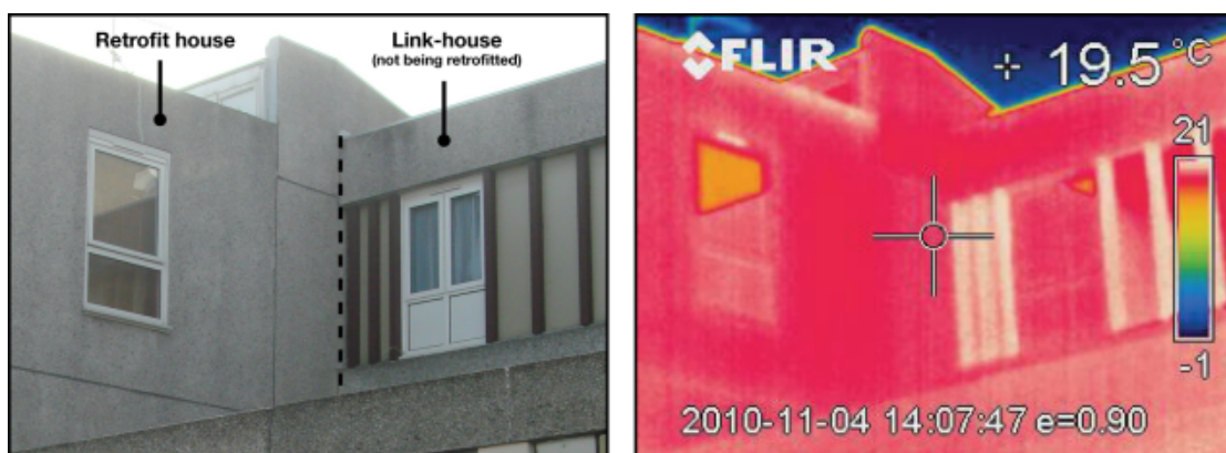
Figure 5.6 Thermal image of the partition wall between the retrofit house and link house.
