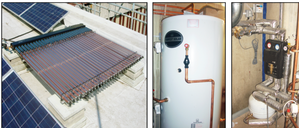
Figure 5.36 Solar thermal collector on the roof and the hot water cylinder in the plant room.
