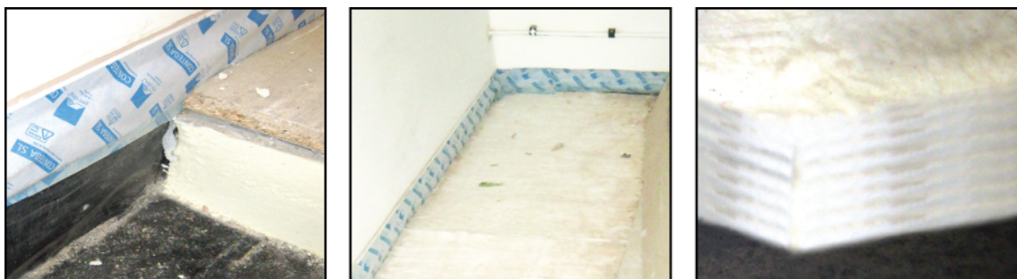
Figure 5.30 Ground floor insulation. PIR in left image. Spacetherm in central & right image.
