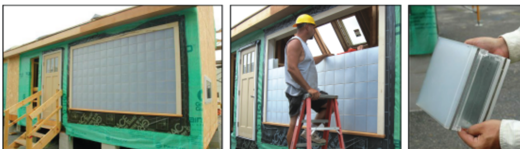
Figure 2.31 The Hunter Douglas Solar Decathlon house incorporating a Trombe wall containing granular aerogel and glass blocks filled with water.
