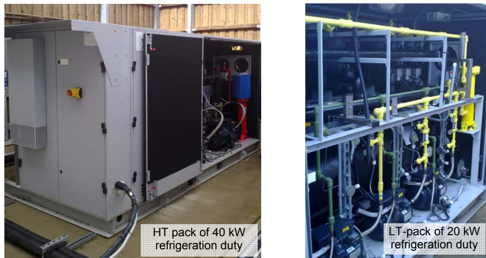
Figure 2.14 Integrated cascade all-CO 2 plant in Tesco Ramsey, UK
