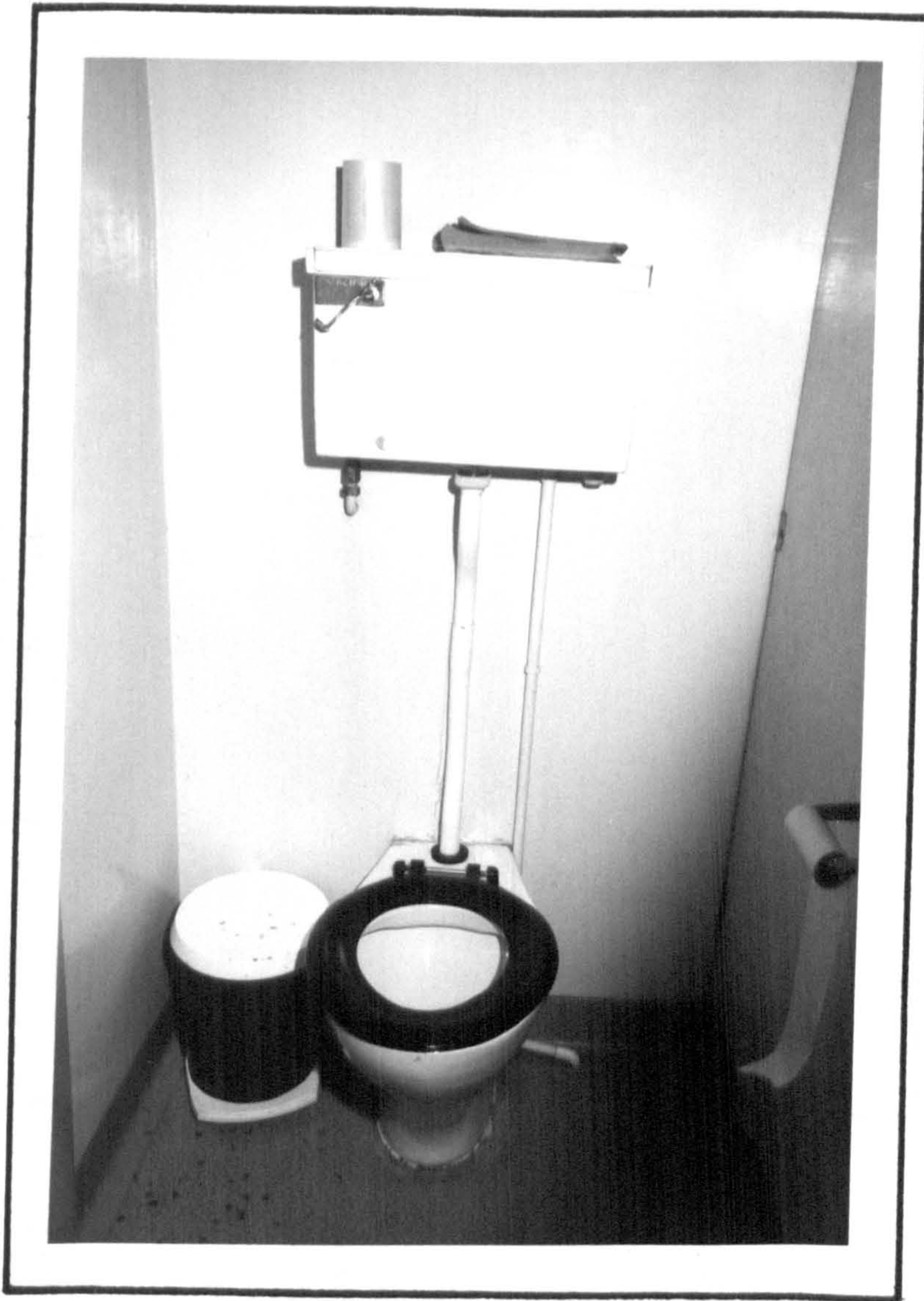
FIGURE 8/12. - Cable to 'Float Switch' in Cistern Concealed inside 15 mm. (I.D.), U.P.V.C. Pipework.
