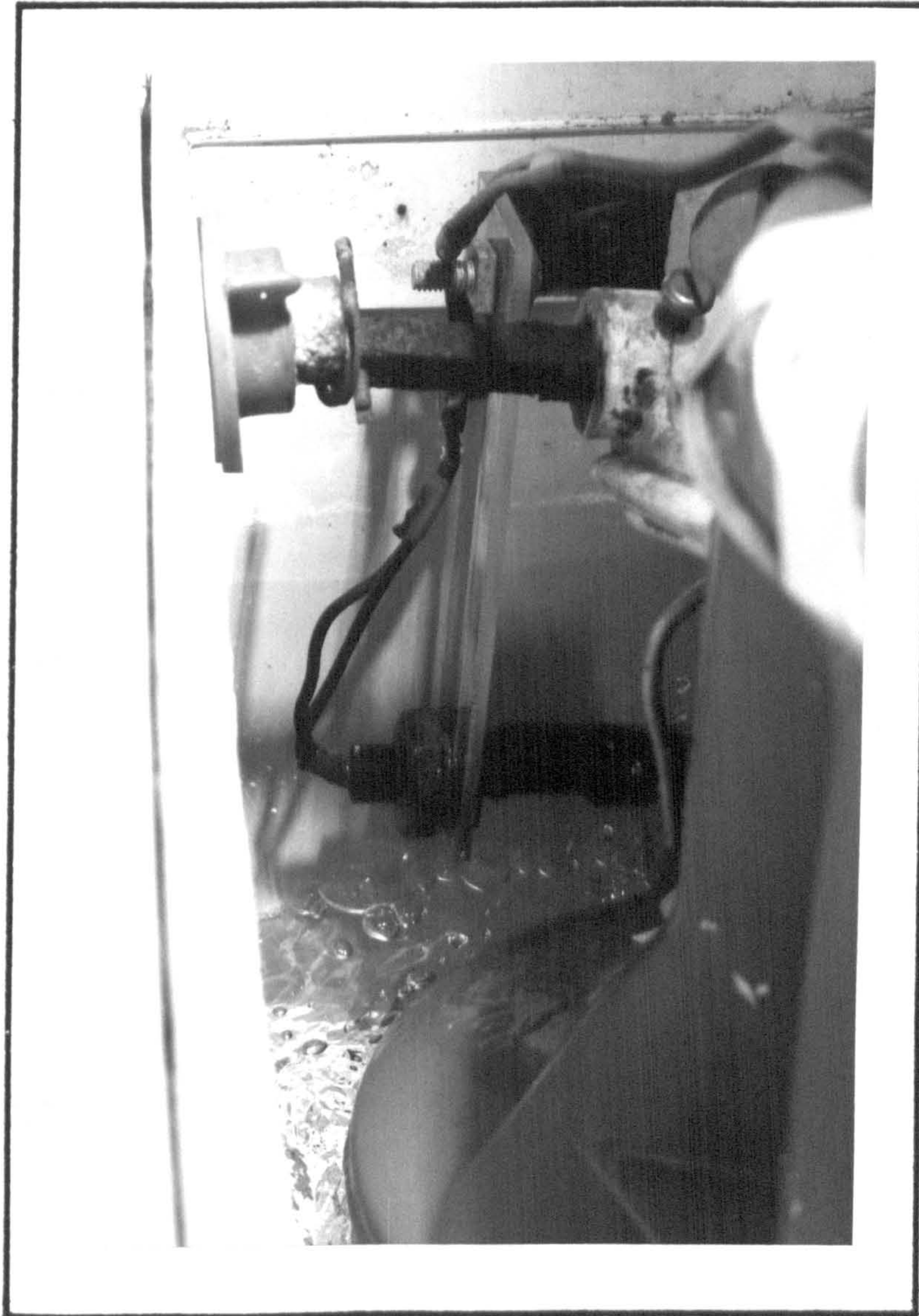
FIGURE 8/10. - Installed 'Float Switch', ('On-Site')
