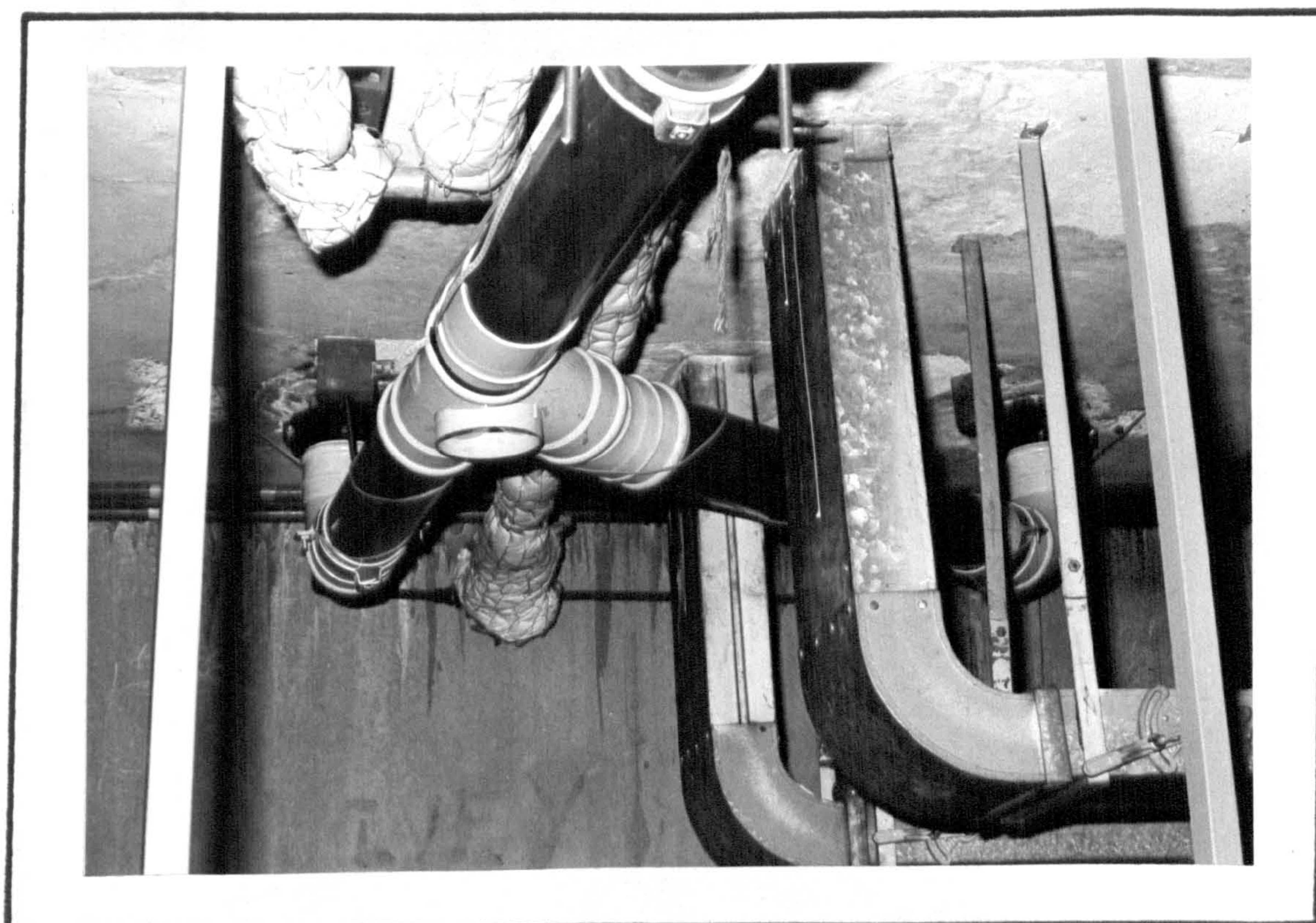
FIGURE 8/2. - Connection of 'Branch-Line' W.C. Pan to Main Straight Length of Monitored Pipework, ('On-Site').
