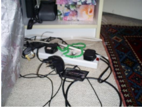
Wires lay on the floor.
