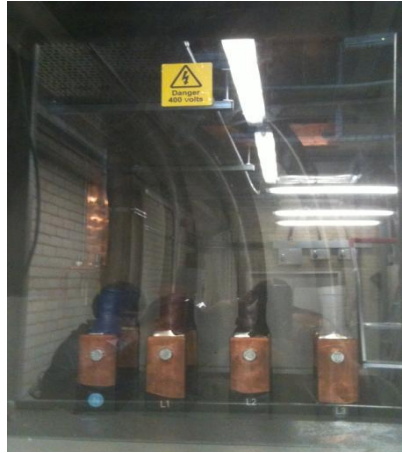
Fig. 3.1 Tower 'A' / Howell building incoming LV breaker (PCC)
