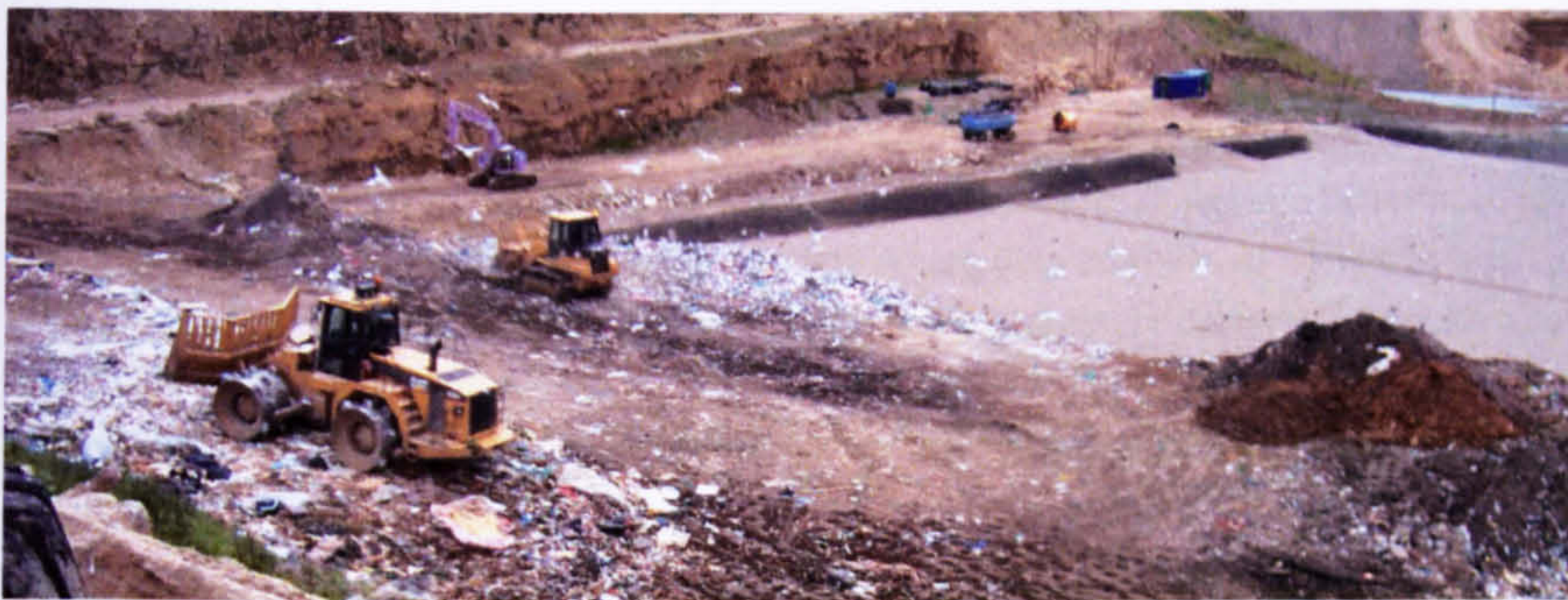
Figure 3 A Landfill site where the waste from Pactiv's compactor bins ends up.
