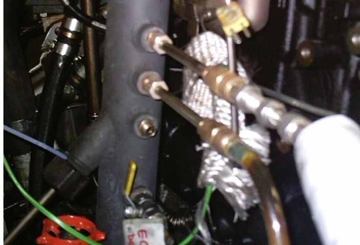
Figure 10 Exhaust downpipe showing sampling ports
