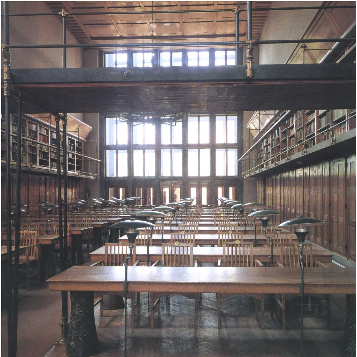
Use of gas piping as handrails and other fittings
