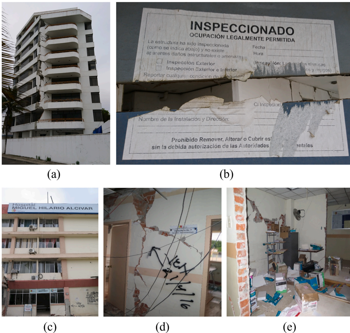
Fig. 1. Photographs of buildings in the city of Bahía de Caráquez, Manabí province, Ecuador, that experienced long seismic downtime after the 2016 Ecuador earthquake: (a) and (b) a residential building with visible structural damage that led to the loss of functionality and issue of inspection tag (photos were taken by the first author in September 2019); (c), (d) and (e) exterior and interior views of the Miguel H. Alcívar hospital building that lost functionality (photos were taken by the second author in May 2016).
