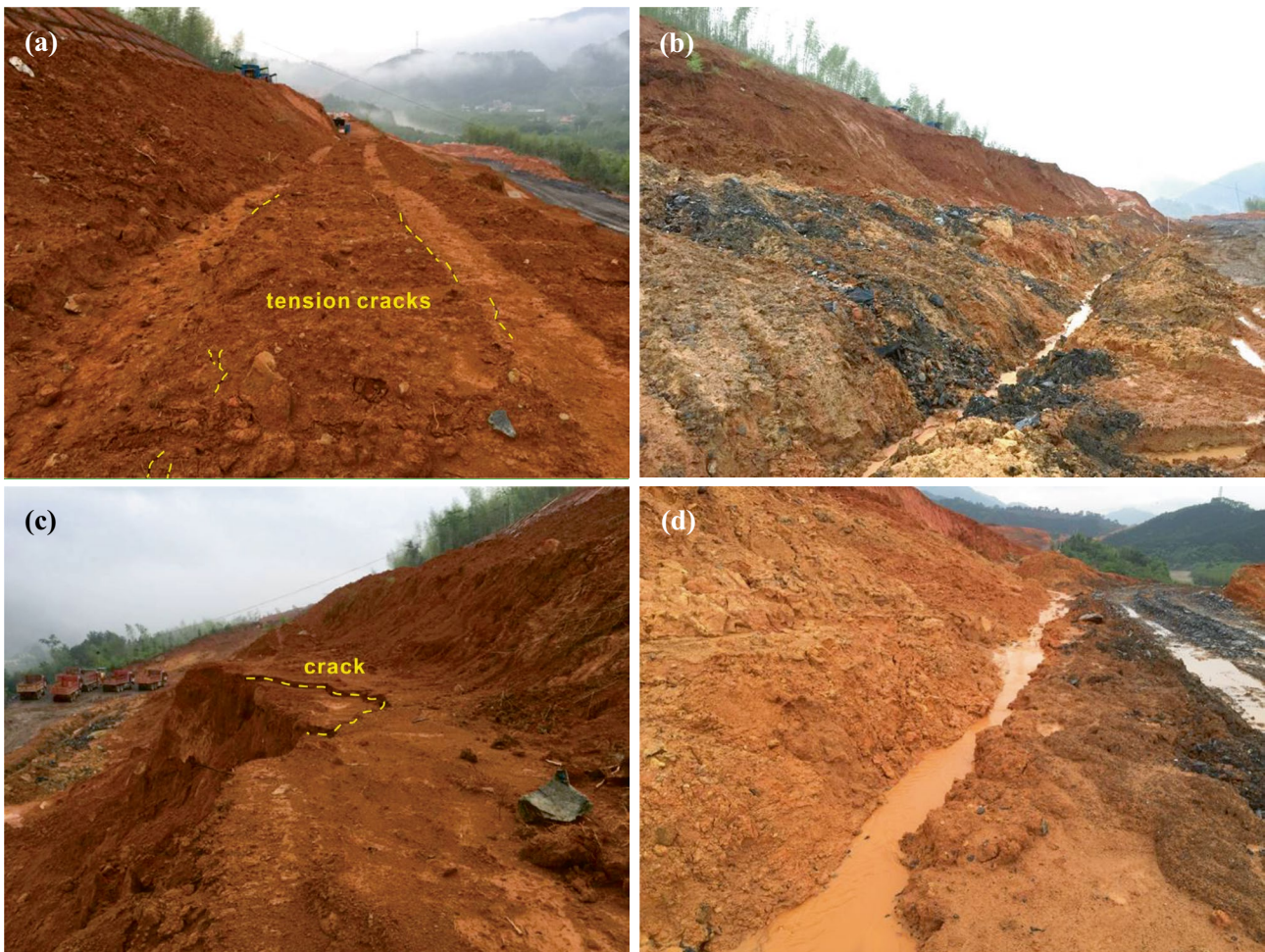
Fig. 6 Deformation and rain seepage of the first slope: a tension cracks (March 2016), b rain seepage at the slope toe (March 2016), c failure pattern (April 2016), and d rain seepage at the slope toe (April 2016)
