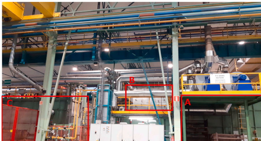
Fig. 12. Photo of the WHR system based on HPHE installed in Fagor Ederlan S. Coop.: a) solution heat treatment furnace; b) HPHE; c) ageing heat treatment furnace.
