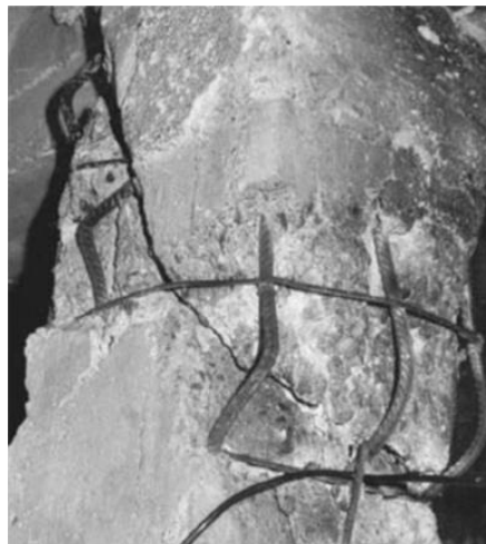
Figure 2-10: Damage to a load bearing reinforced concrete column following a fire, leaving the steel exposed (Venanzi, et al., 2008)
