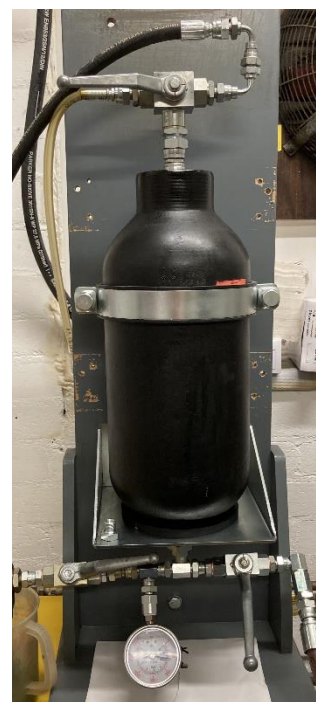
Figure 3.4 Fuel pressure vessel (tank)
