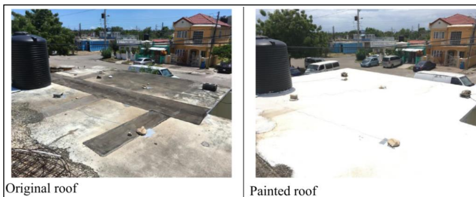
Figure A-1: Application of cool roof paint on the roof of Portmore, Jamaica case study house. The cool roof paint application was carried out by research partner at the University of Technology, Kingston, Jamaica.
