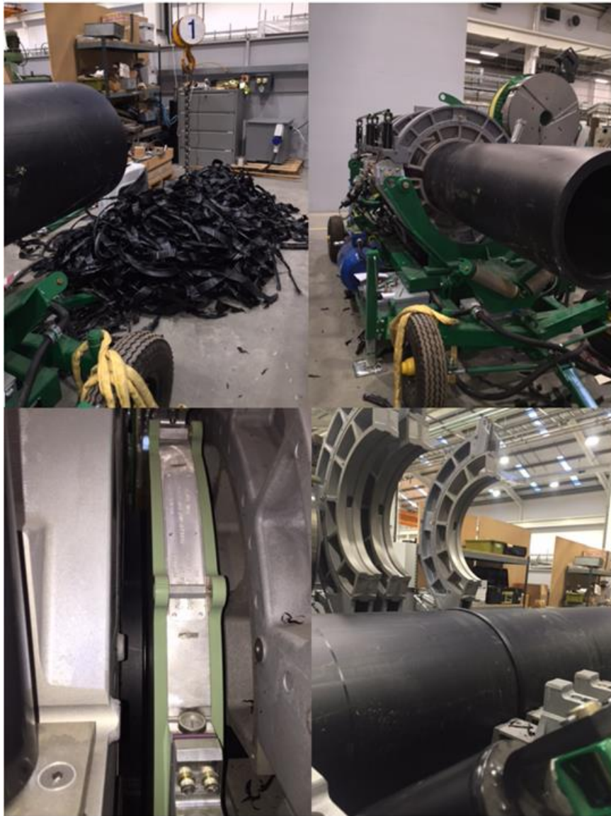
Figure 6-30, From top left clockwise, Trimming, pipe position in the machine, heater plate in place, final weld
