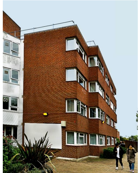
Figure 5: A view of the student accommodation façade that was insulated with VIPs at Brunel University London (UK).
