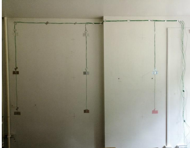
Figure 7: Thermocouple locations on the inner surface of wall inside the room.
