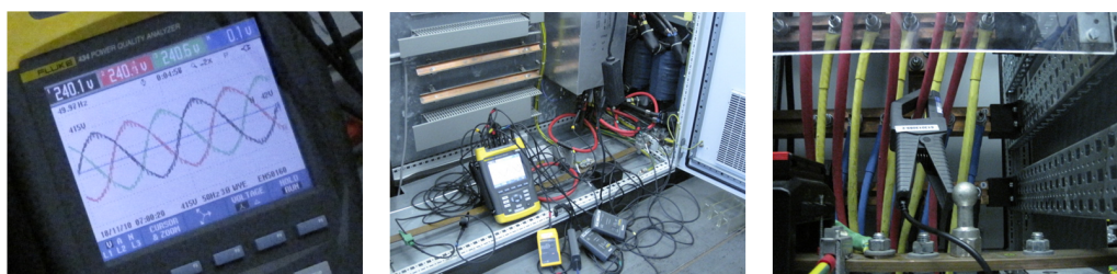
Figure 4.6: Power Quality Analyser Loggers with Clamp CT's and Flexible Voltage Probes
