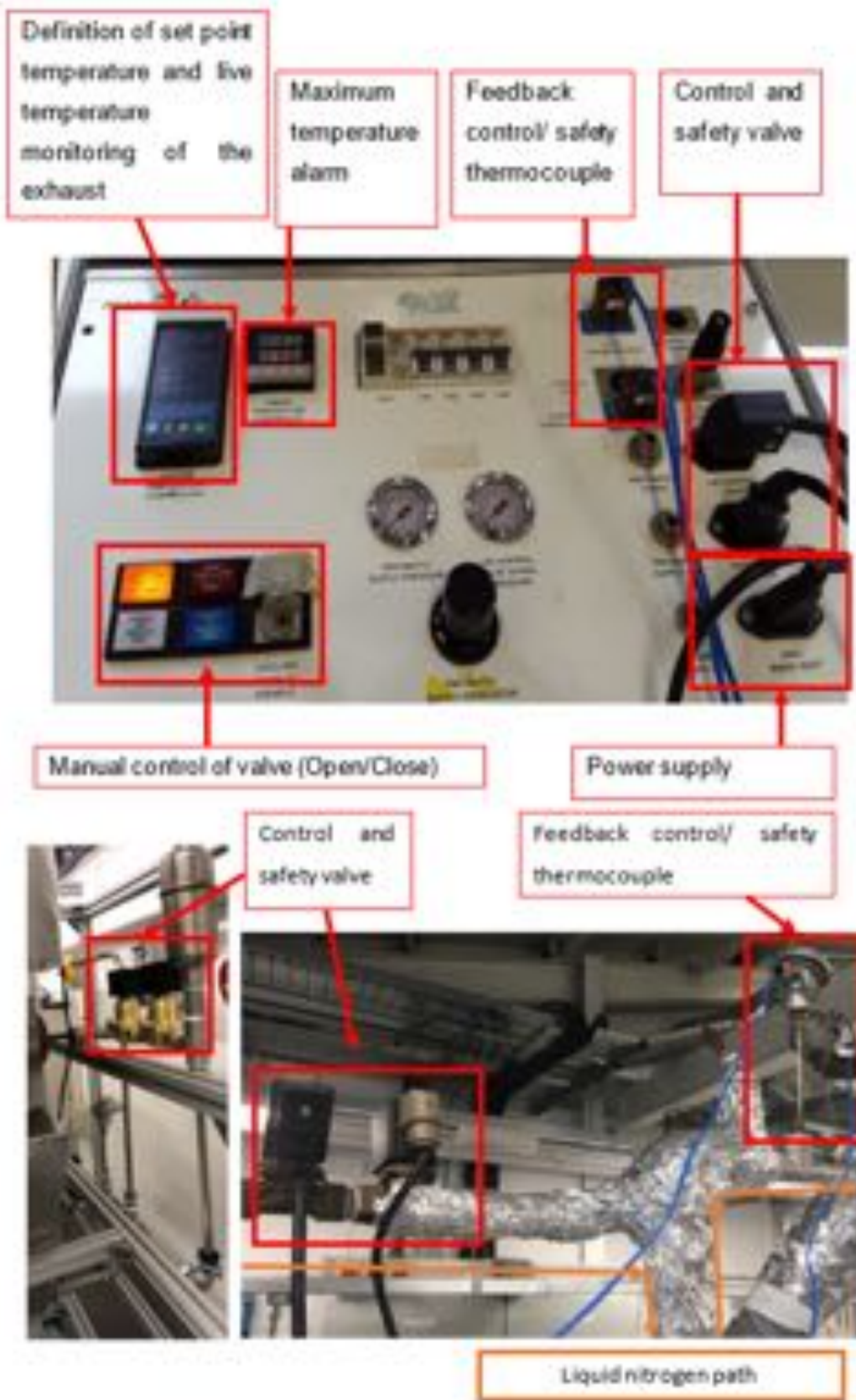
Figure 5-13: Liquid nitrogen feed controller
