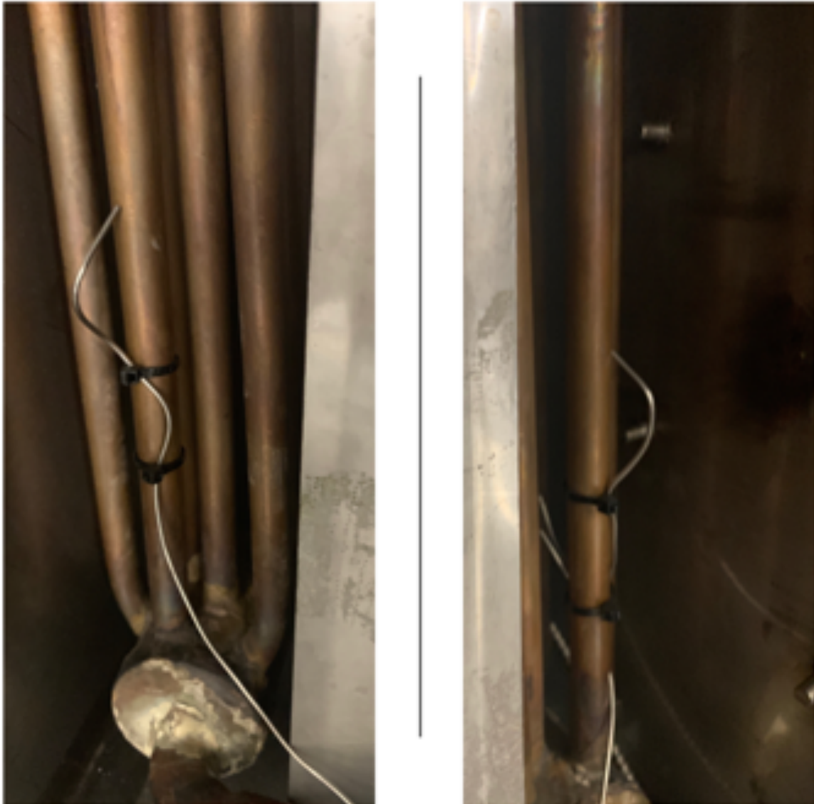
Figure 5-15: Thermocouples to monitor heat pipe temperature
