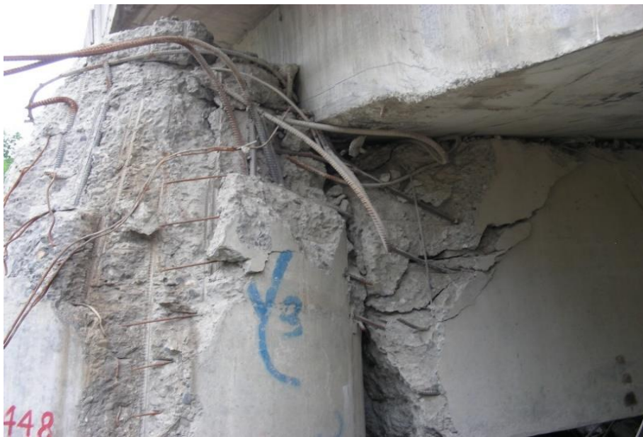
Figure 1.2 Damaged RC bridge pier during the Wenchuan Earthquake in 2008 (Yen et al. 2011)
