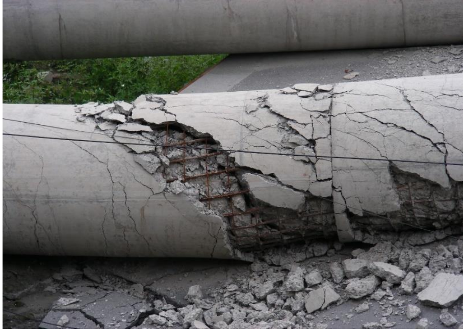
Figure 1.1 Collapsed RC bridge pier during the Wenchuan Earthquake in 2008 (Yen et al. 2011)
