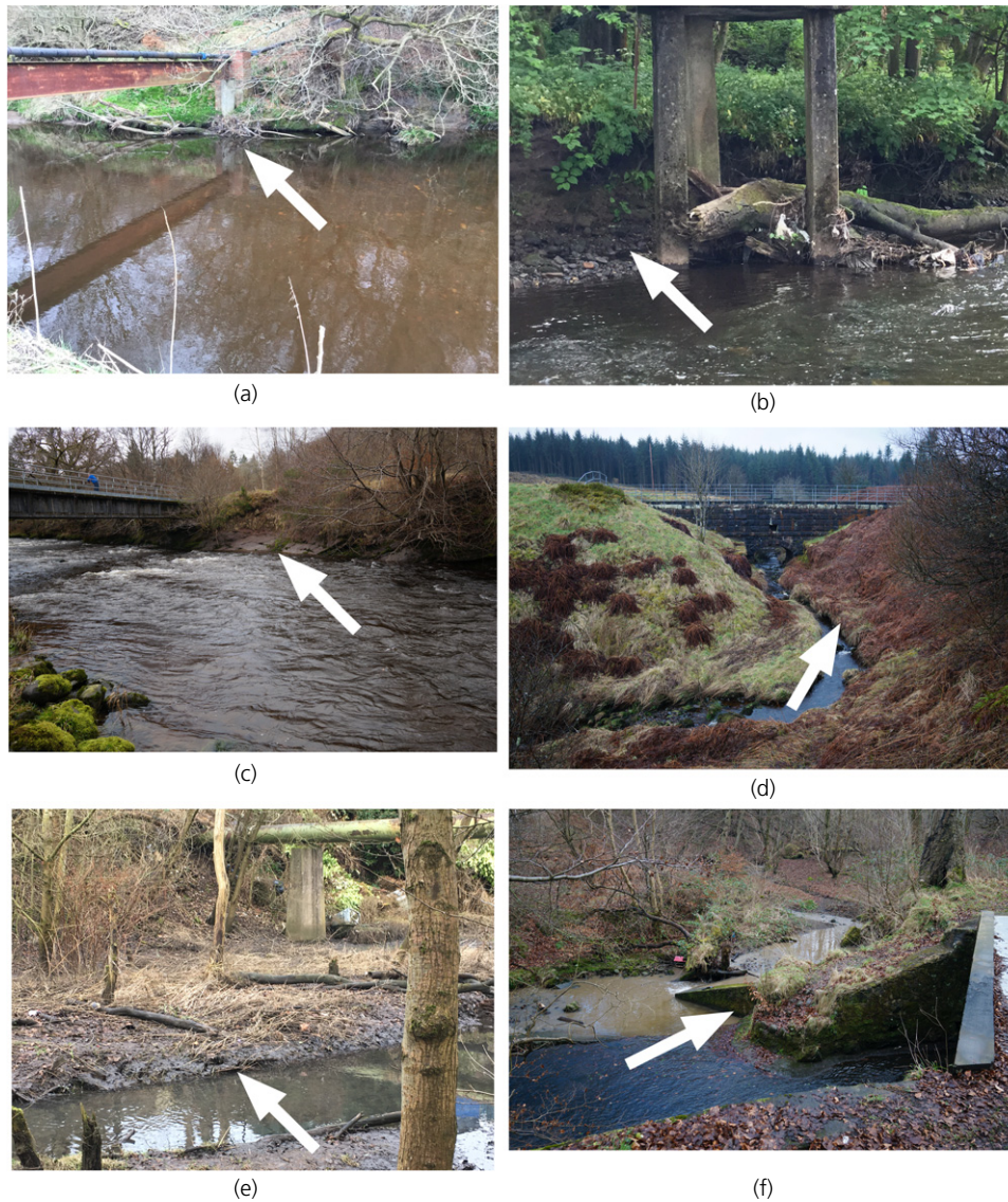
Figure 1. Example of geomorphological factors affecting bank stability. White arrows point to specific features: (a) bank undercut close to pipe crossing abutment; (b) and (c) bank erosion close to pipe crossing pier and abutment; (d) very steep banks close to crossing; (e) highly erodible material close to crossing pier; (f) undermined bank protection integrated into the crossing abutment construction
