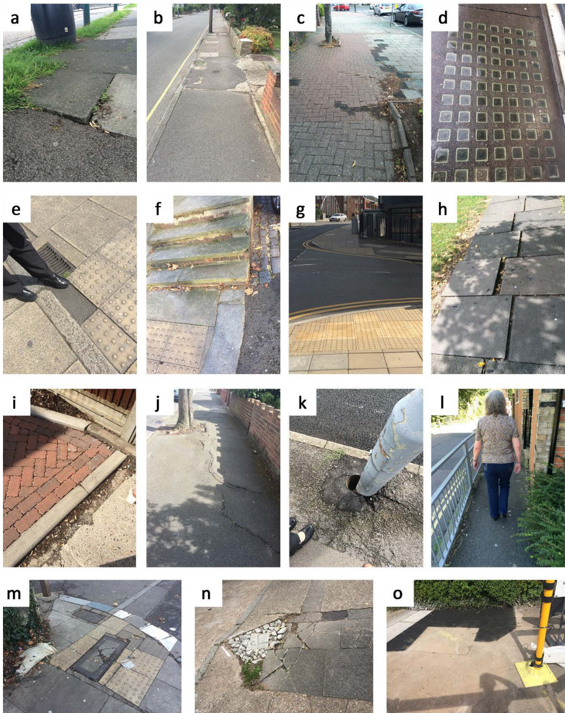
Figure 4-7. Poor pavement conditions photographed in London.
