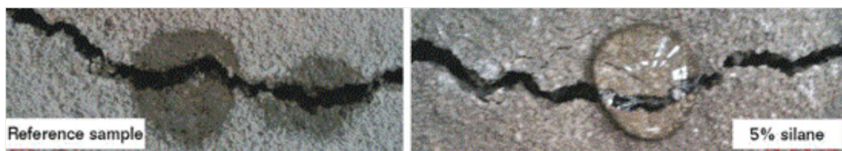
Figure 2-11 - The difference between untreated concrete and concrete treated with silane after the initiation of cracks (Jiesheng et al. 2018)
