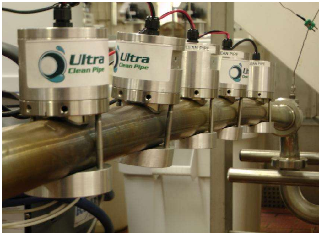
Figure 8.16. HPT transducers attached with low acoustic attenuation couplant silicone and UCP support clamped to a 1.5 m pipe for the field trials for the non-flow experimentation.
