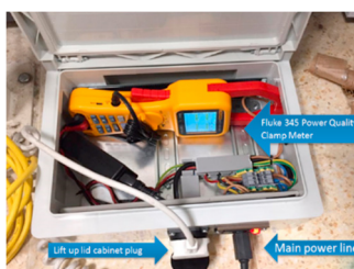
Fig. 4. Energy consumption metering box.
