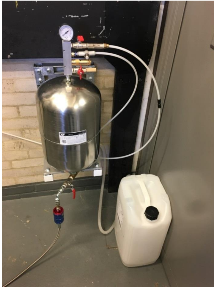
Figure 3-11 Pressurized water tank and some other components of the water injection system in the test cell
