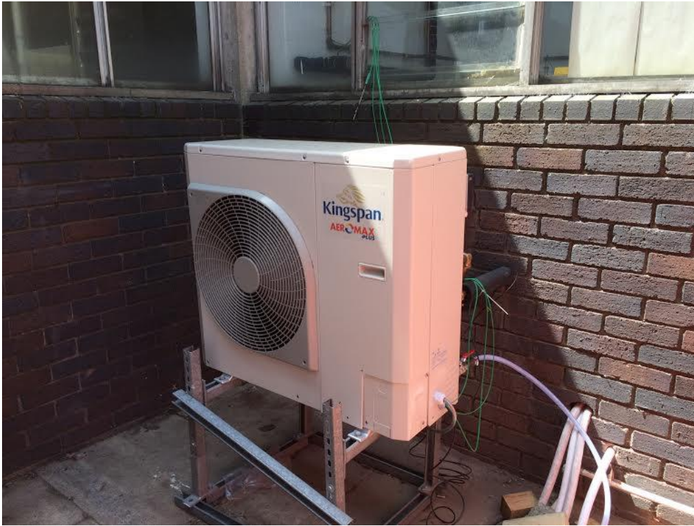
Figure 3. 2 Air-source heat pump
