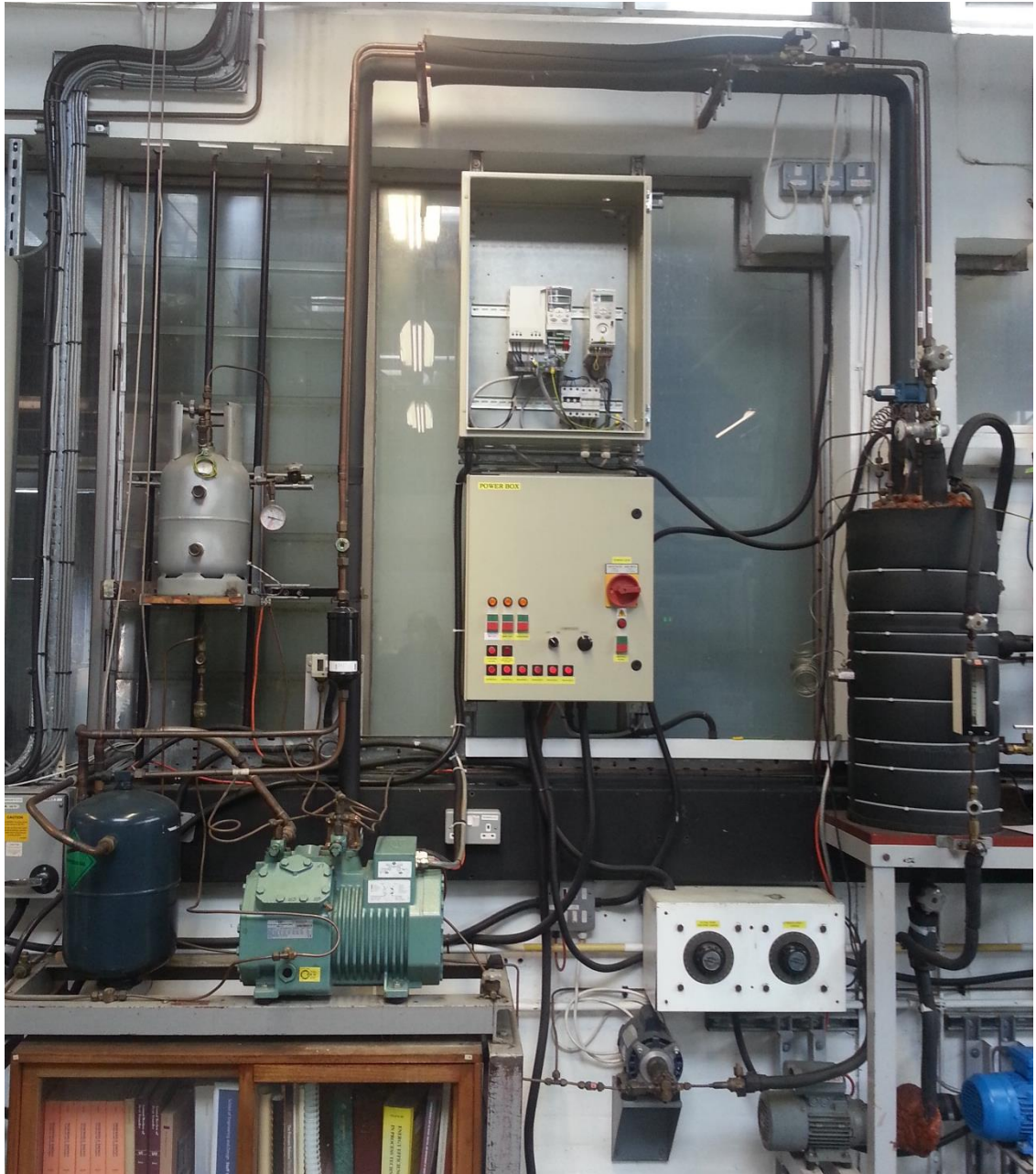
Figure 3.4 Photograph of the external cooling system.
