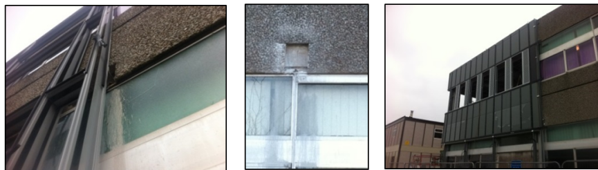
FIGURE 3.7: External retrofit glazing module build up. (reproduced courtesy of Henry J Lyons Architects)
