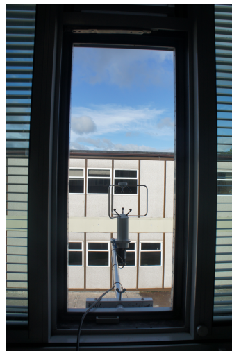
FIGURE 3.18: Plain Opening in retrofit space used for comparing with slotted louvre. The existing individual louvre sections normally screwed into the facade frame (see figure 3.9) were removed and replaced with a single mock up louvre shown in Figure 3.19
