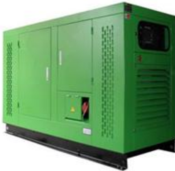
Figure 5.9: Examples of central generators used in Saudi Arabia for remote villages ( https://www.google.com/imghp )
