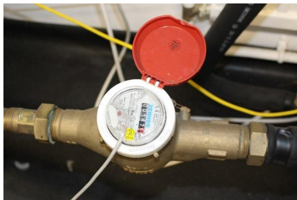
Figure 3.21. pulsed screwed flow meter
