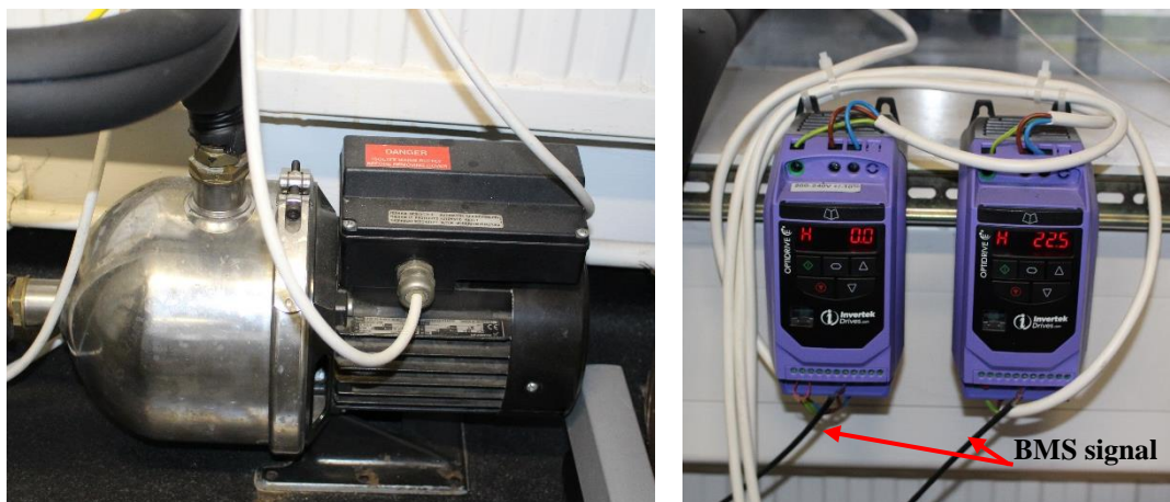
Figure 3.17. Motor driven pump with a digital inverter
