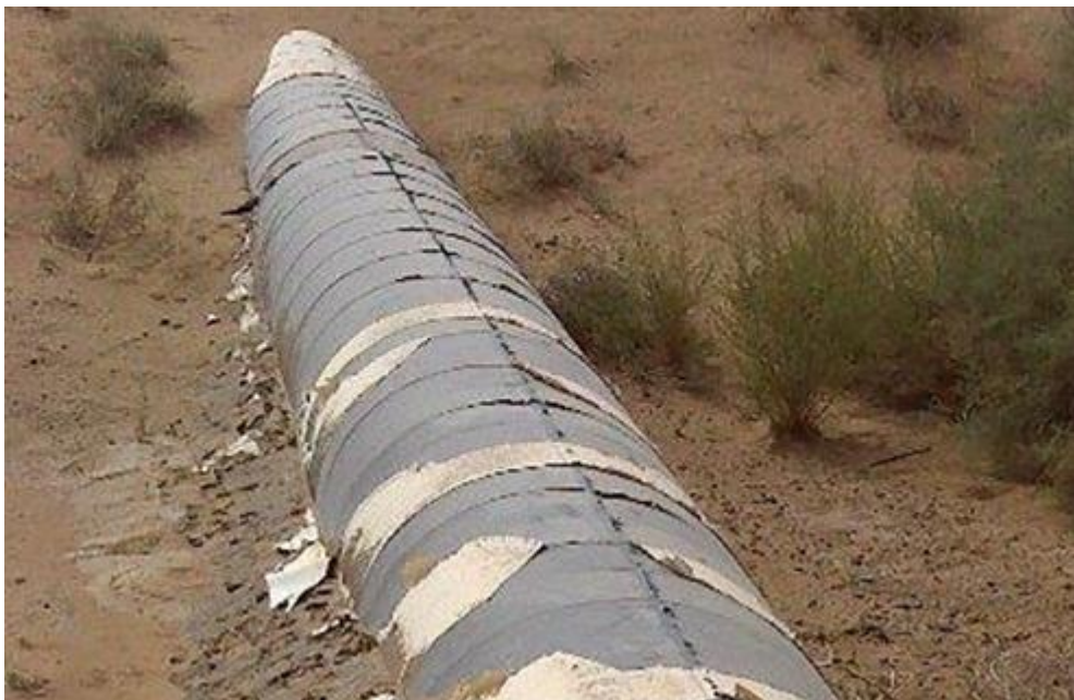
Figure 3-16. Example of pipeline exposed due to soil erosion.
