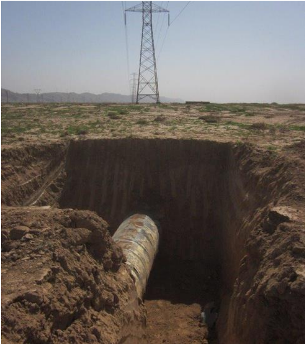
Figure 3-14. Example of pipeline close to AC power lines.
