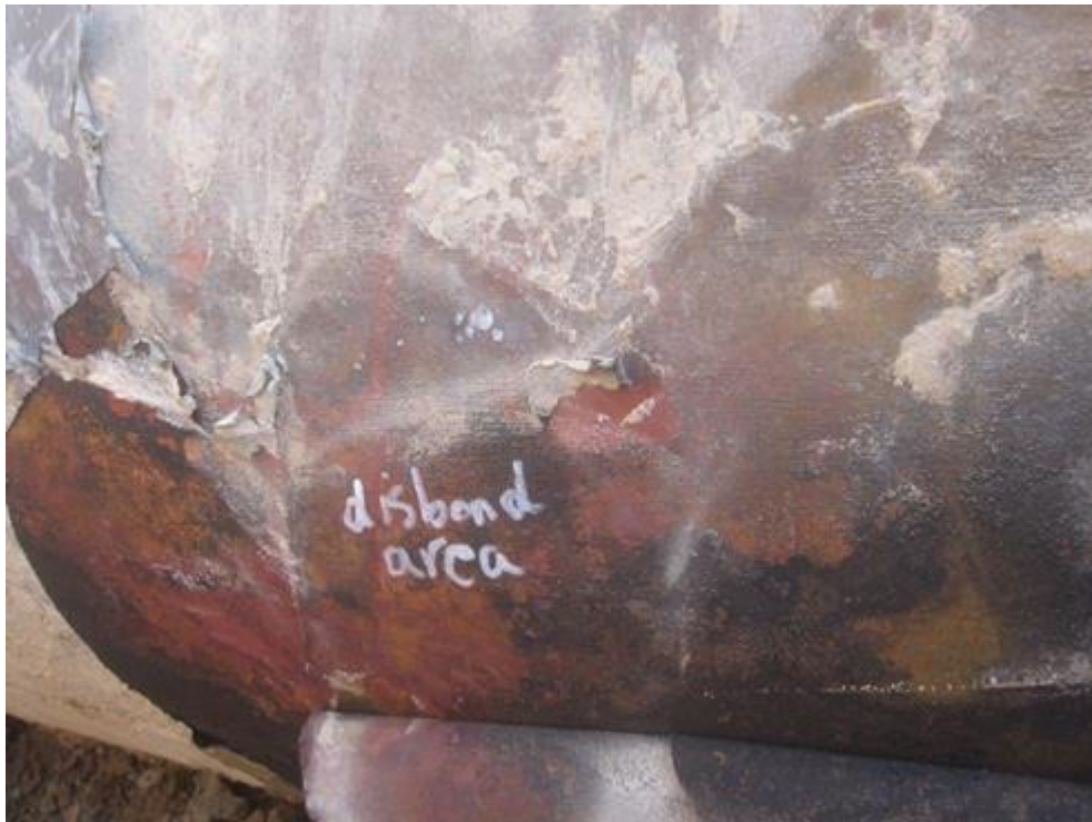
Figure 3-17. Example of disbonded coating next to damaged coating.
