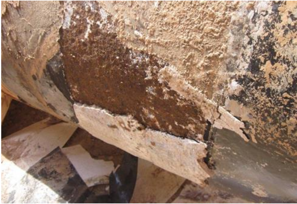
Figure 3-8. Example of scale covering exposed and corroded area of a pipeline.
