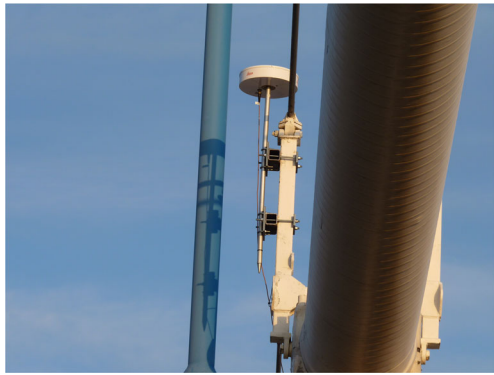
Fig. 7 Antenna located on the suspension cable
