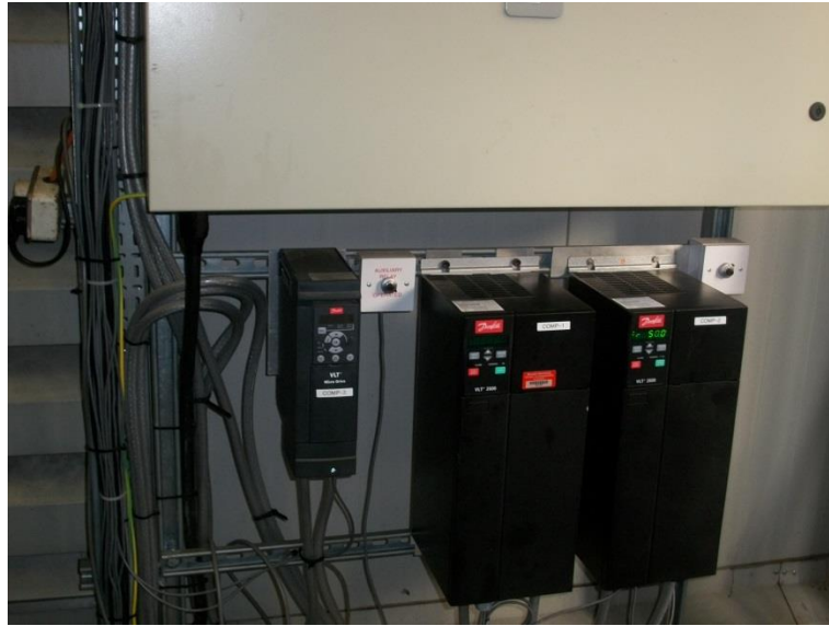
Figure 5.8 Compressor variable speed controllers
