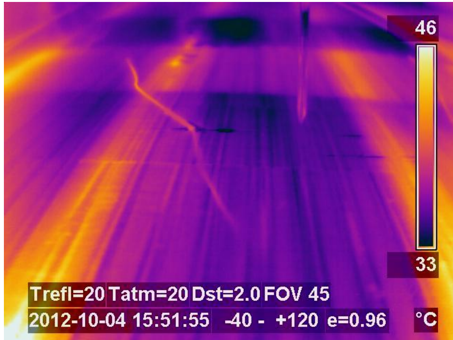
Figure 7.6 Thermal imaging capture
