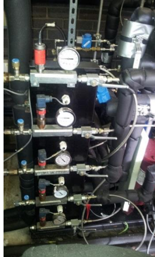
Figure 5.27 Pressure gauge used on the CO 2 system
