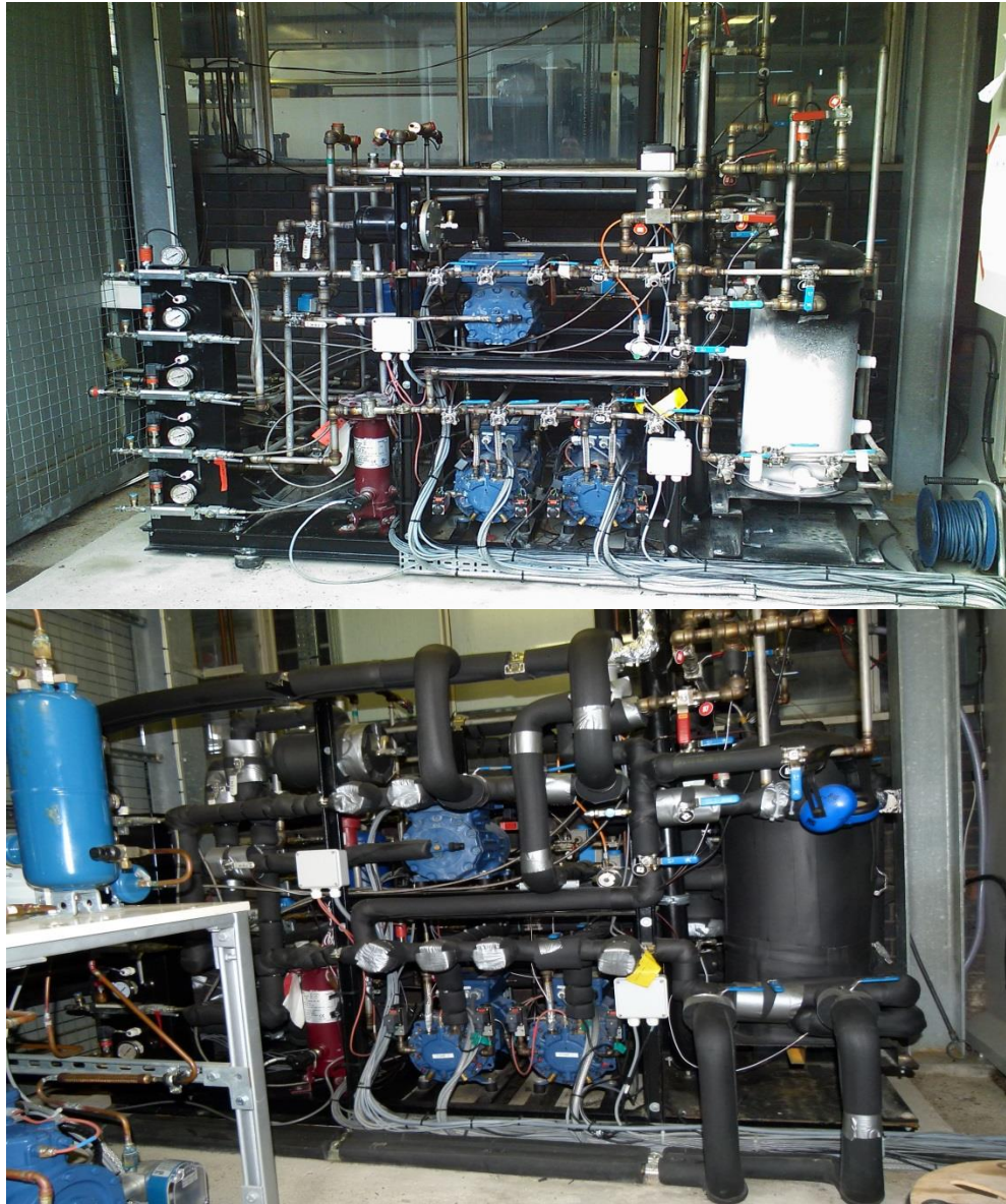
Figure 5.2 CO 2 booster experimental test rig
