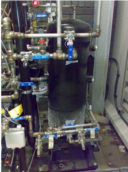
Figure 5.17 Liquid receiver installed in CO 2 system
