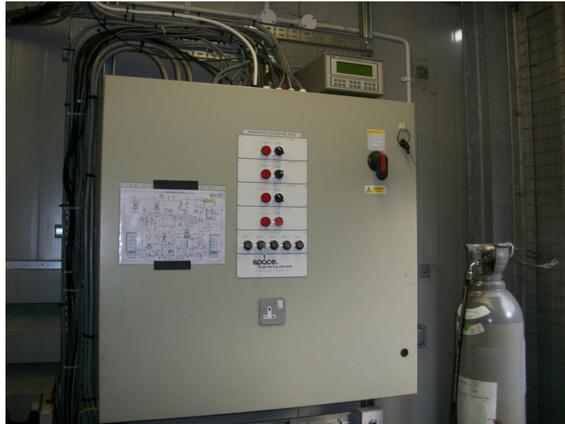
Figure 5.34 CO 2 booster control panel
