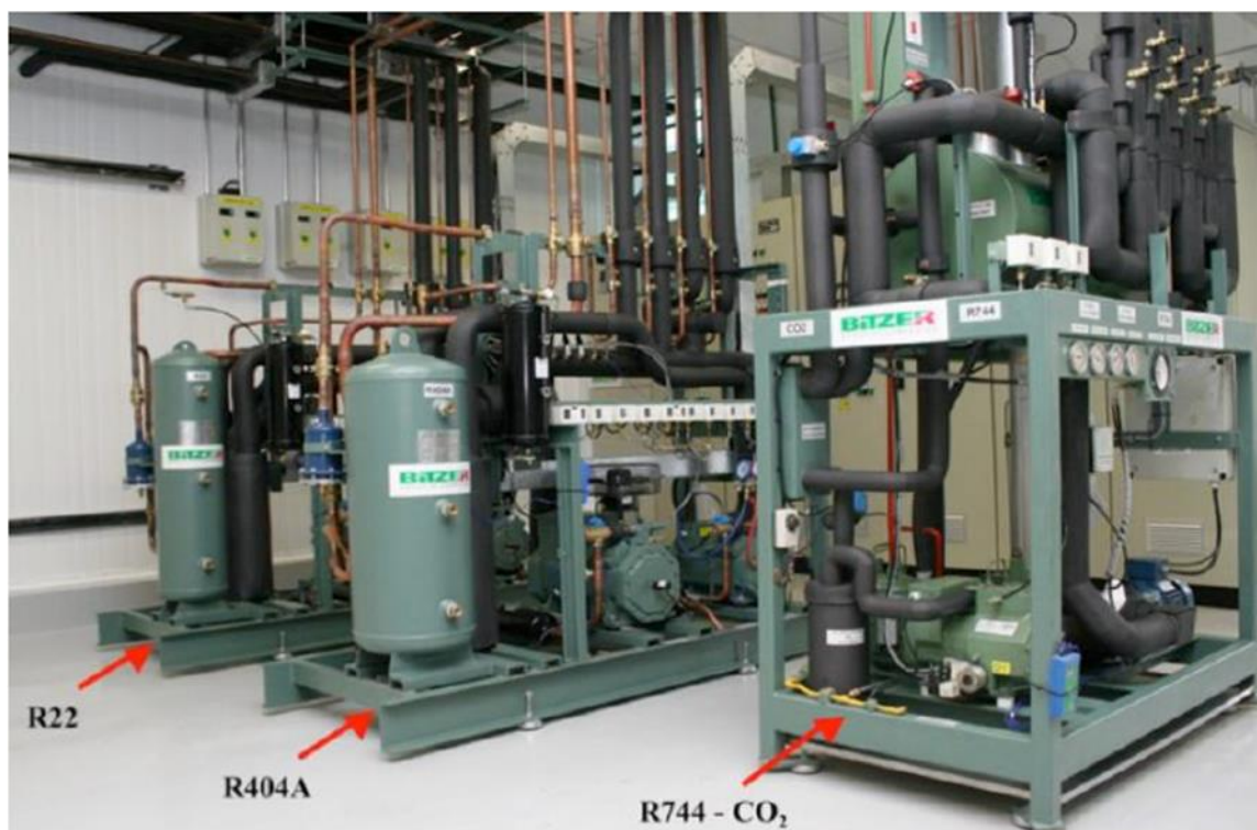
Figure 3.11 R22, R404A and CO 2 /R404A refrigeration systems trailed by BITZER for supermarket application
