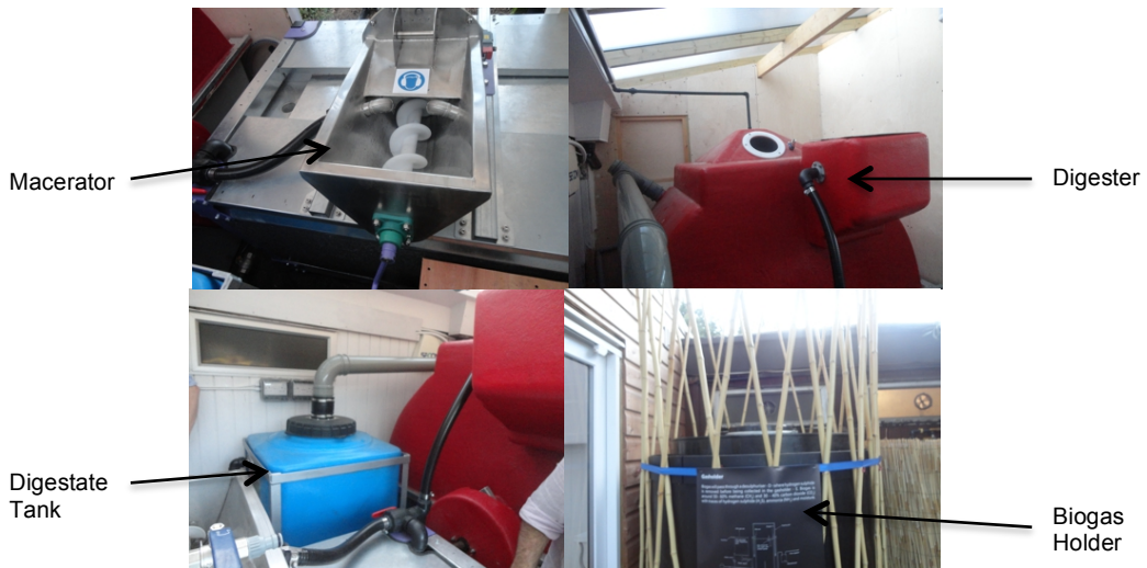
Figure 3–9 Camley Anaerobic Digester system showing macerator, bio-digester, digestate tank and biogas holder.
