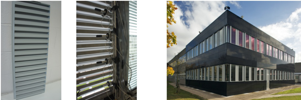
Figure 1: Left: Louvre module used for testing. Middle: louvre opening. Right: External facade of the testbed building showing the pre and post retrofit (see http://www.zero2020energy.com for more details). Integrated vertical slotted louvre banks also visible
