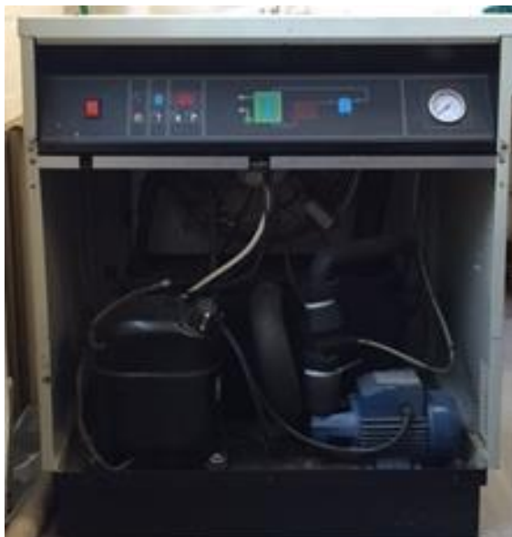
Figure 3.6 Photograph of the chiller unit.
