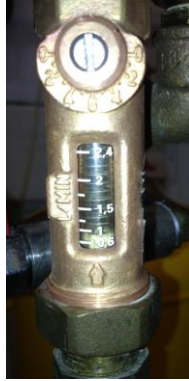
Figure 3-11. Float type flow meter that controls the TGM heat exchanger.
