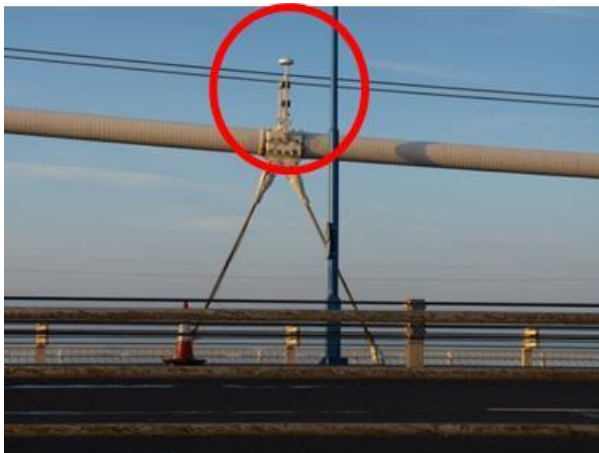
Figure 8, A GNSS antenna located on the Severn Suspension Bridge's suspension cable, Location C.
