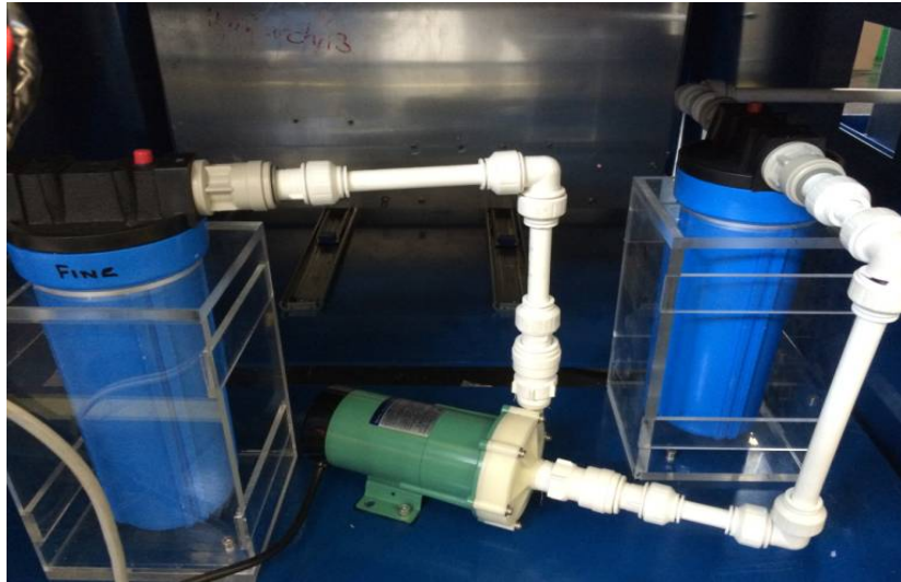
Figure 5-19: Picture of the 2 filters and the pump
